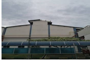
Phase 3 Building - Roof Flied Off
