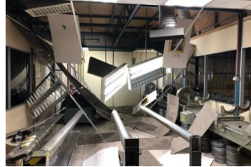
D&E Section - Ceiling Ducts Collapsed
