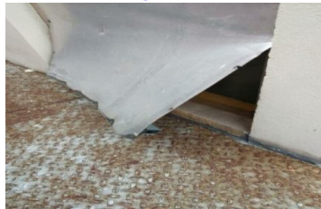
WTM Building - Loosen Roof Flashing
