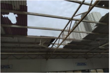
Sri Murni Surau & Kitchen - Broken Roofs
