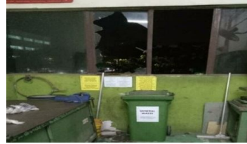
Maintenance Room - Broken Glass
