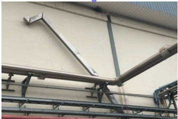
Phase 1 Building - Rain Gutter Broken and Flied Off
